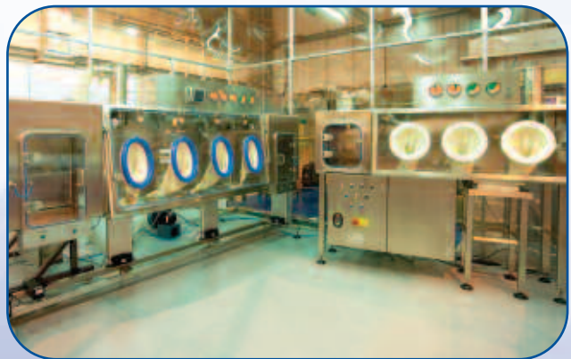
Isolators in Test Area
