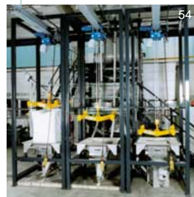
Plant for fibre dosing
