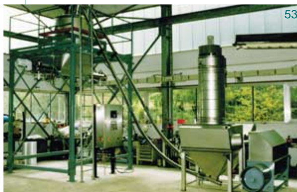
Sugar dosing plant in the drinks industry
