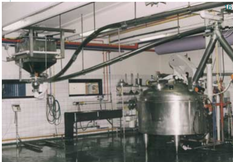
Weighing and conveying plant for sugar
