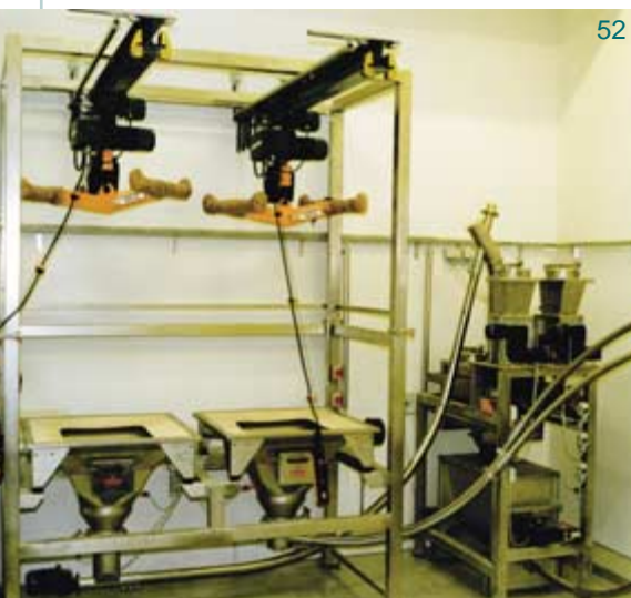
Dosing and mixing plant for liquorice production
