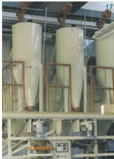
EMDE-LIFT in a high-precision dosing plant for synthetic resin and aluminium powder
