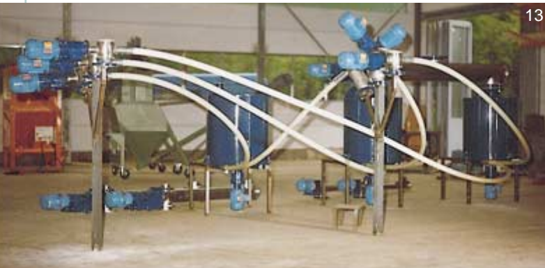
Additive dosing with EMDE-LIFT for the petrochemicals industry
