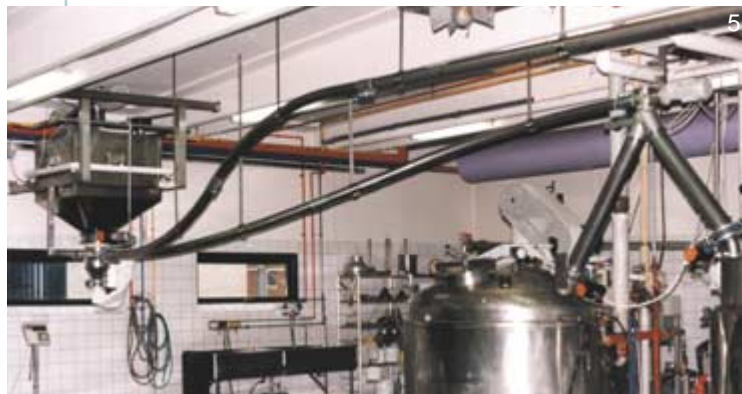
Two EMDE-LIFT MDB 80 conveying sugar
